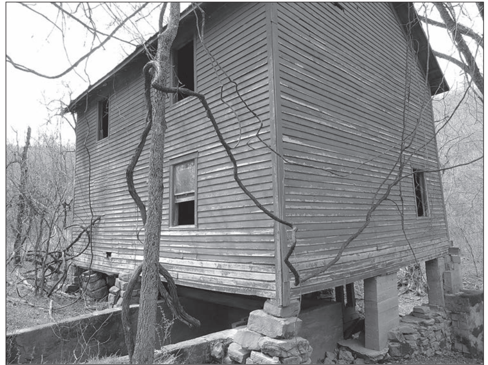
The grist mill at Hazelton Spring, built circa 1885, as it appeared in 2016. The field stone foundation has been reinforced in places with concrete piers. In the lower left of the picture is the top of the fore bay where spring water was directed into a deep hole housing the vaned turbine. The vertical turbine shaft turned a series of gears and belts which operated the grist mill. A belt from the turbine also turned a shaft that operated the nearby sawmill, which is no longer present. The water generated enough power to operate the grist and saw mills simultaneously.
